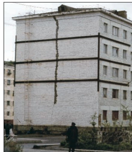
Oops. When Siberian permafrost thaws, buildings can lose their footing and slowly crumble.
